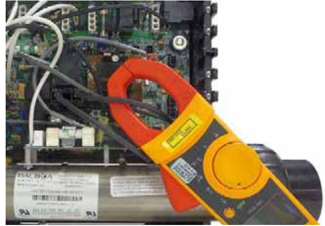
AMPERAGE HEATER TEST BP2100G1
