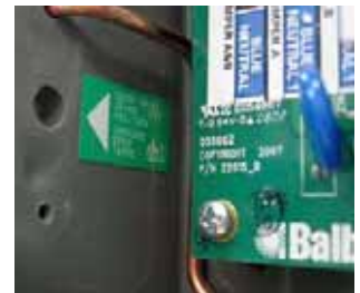
Ground in System Enclosure
